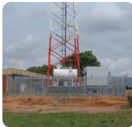
AD9090H TOWER ON QUICKSITE GRILLAGE BASE
