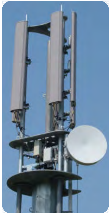
TYPICAL LOADING ON 2-USER MONOPOLE: SECTORS, DISHES & AMPLIFIER UNITS
