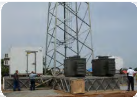
QUICKSITE GRILLAGE BASE WITH TOWER & TYPICAL EQUIPMENT IN POSITION FENCING NOT SHOWN
