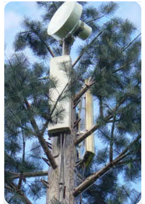
ANTENNAS IN `FOLIAGE` GREEN/BROWN COLOURED ANTENNA OPTION AVAILABLE TO MINIMISE VISUAL IMPACT
